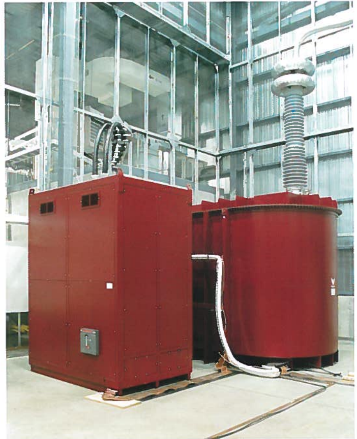
350kV, 700KVA Tank Type Transformer used for testing icing conditions on power network components.
